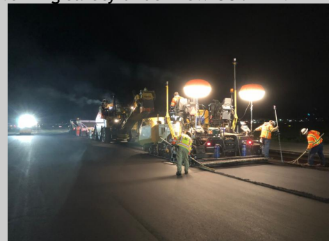
A pre-COVID-19 paving operation on the state highway system. Caltrans is considering converting some night work to daylight hours due to the greatly reduced traffic
